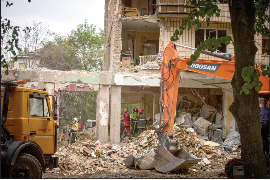
EFREM LUKATSKY/AP PHOTO Ukrainian Emergency Service work on the site of Russia's Tuesday deadly missile attack that ruined a multi-story residential building in Kyiv, Ukraine, Wednesday, June 18, 2025.
